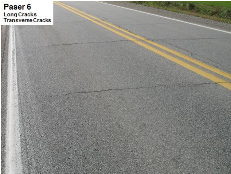
Paser 6 Block Cracking Starting Sealed Transverse Cracks
